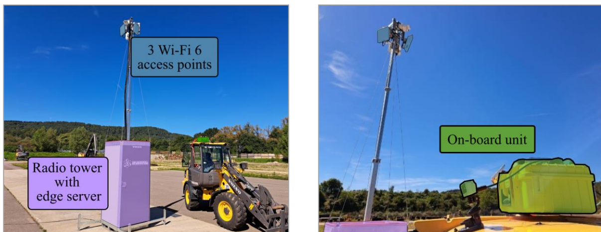
Figure 2: Radio tower with edge server (left) and construction machine with an on-board unit (right)
